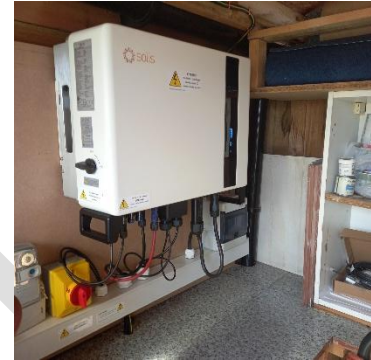
Figure 15: PV Battery storage installed thanks to the CIG.
